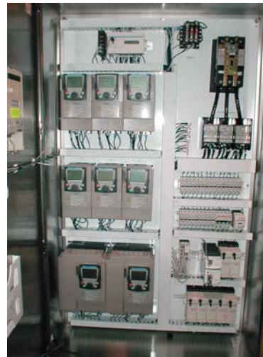
An Industrial Control Panel
